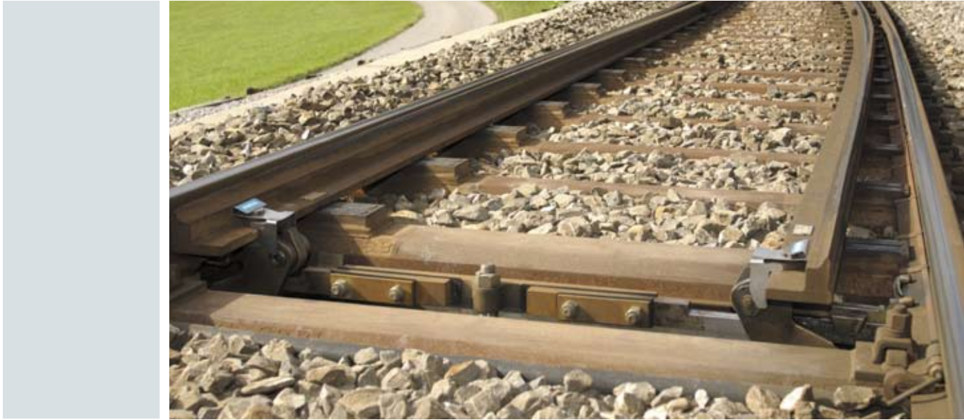
Pawl point lock installed in switch.
